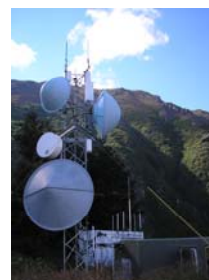
The ALMR Asset Manager completed inventory of Air Force and Army assets at 50 locations this summer, including this site at Hope.
